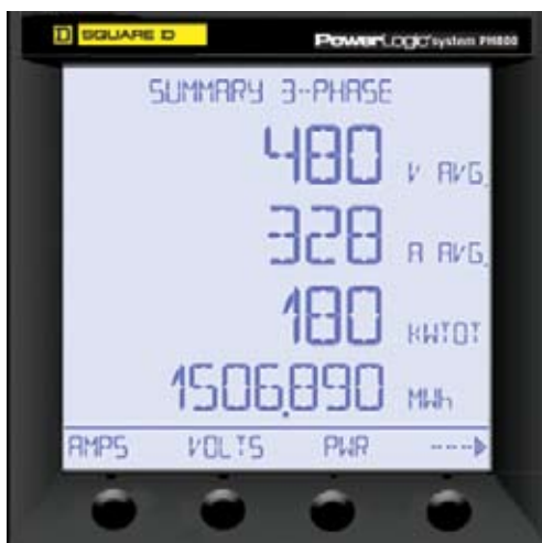
Front panel display showing function selection buttons and 3-phase voltage, current and power summary display.
