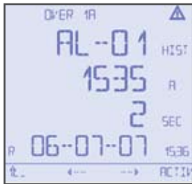
Alarm display showing active alarm
